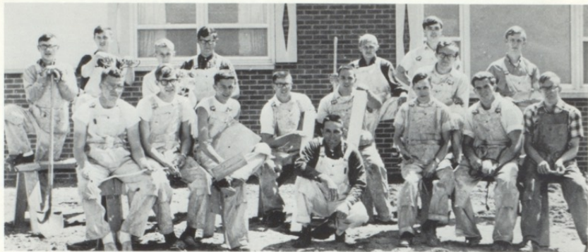
HOUSE CONSTRUCTION CREW: Sitting left to right—G. Easterday, M. McKay, D. Waite, D. Wilkins, J. Lewis, L. McLaughlin, B. Pifer, D. Slaton. Standing—L. Rousch, B. Murfin, R. Norton, L. Cornish, B. Synder, F. Johnston, J. Tabor. Kneeling in Front—Advisor, Austin Miller
