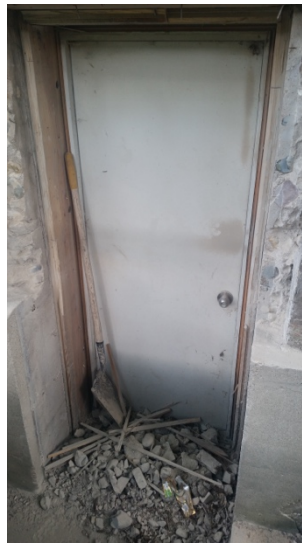
Quincy backside/west old basement entrance; sealed up from inside when elevator was installed in 2000.
