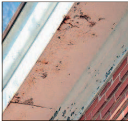
The rusting eaves and enclosed gutters on the Quincy library will be restored. DON REID PHOTO
