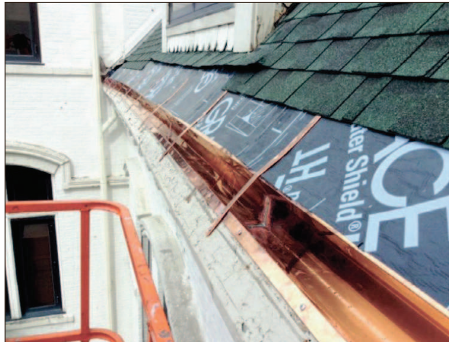
New copper gutters installed into the roof of the Coldwater Library, along with repairs to the shingles and flashing, should prevent further roof leaks. DON REID
