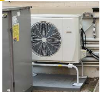
Server Room Air Conditioner
