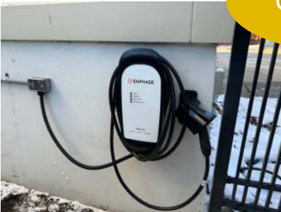
Charger for Upcoming Bookmobile (Diesel vehicle has a battery instead of a generator for interior electrical.)
